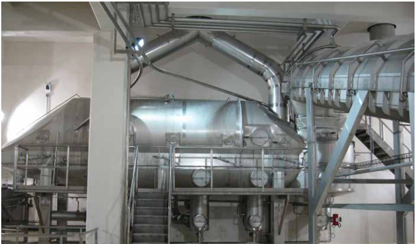
A section of a dairy drying system - a fluid bed and a crystallization conveyor
